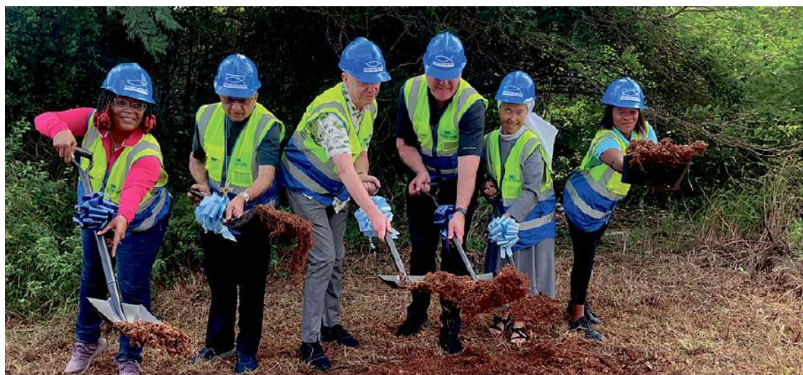
Food For The Poor (FFTP), in partnership with Entrepreneurs Across Borders (EAB) and the UpMobility Foundation, broke ground in December 2024 for the Zion Entrepreneurial Village, a sustainable community development project in Martha Brae, Jamaica. Participants in the ceremonial dig included (left to right) Kivette Silvera, then-Executive Director of FFTP-Jamaica; Bishop John Persaud, Apostolic Administrator of the Montego Bay Diocese of the Roman Catholic Church; Martin Babinec, a Silicon Valley entrepreneur and founder of both EAB and the UpMobility Foundation; Ed Raine, President/CEO of FFTP; Sister John Kim, of the Kkottongnae Brothers and Sisters of Jesus, of South Korea; and Tamika Plummer, President of the Zion Community Action Group Benevolent Society. (Photo/Food For The Poor)
